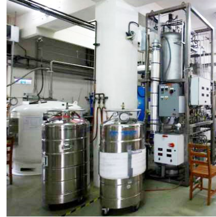
He liquefaction facility
